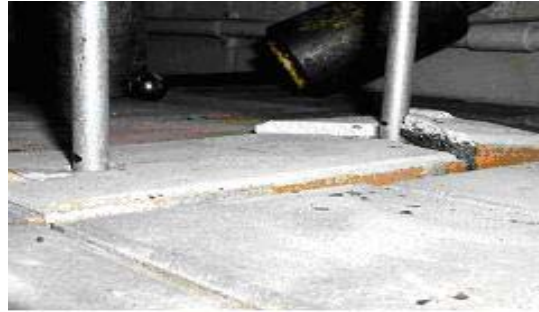
FIGURE 6 - Pullout test – Showing mode of failure
